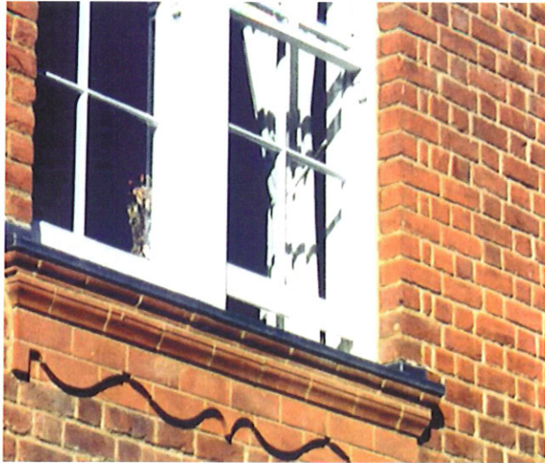
Brickwork cleaned and repointed in 1:2:9 mix, brushed back. Brick detailing well protected and finely pointed.
