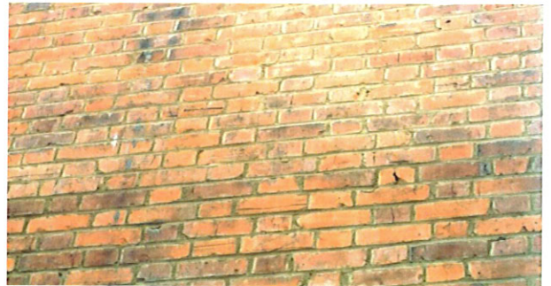
Ten percent patched with second hand bricks and fully repointed in 1:2:9 mix, lightly brushed
