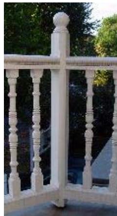
A typical front balustrade on an angled bay. The tapered newel post at the 45degree corner is kept clear of the roof finish on a metal dowel.
