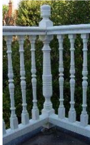
A typical rear balustrade that has been "stretched to comply with Building Regulations. The newel post is kept clear of the asphalt roof finish on a specially made galvanised steel base.
